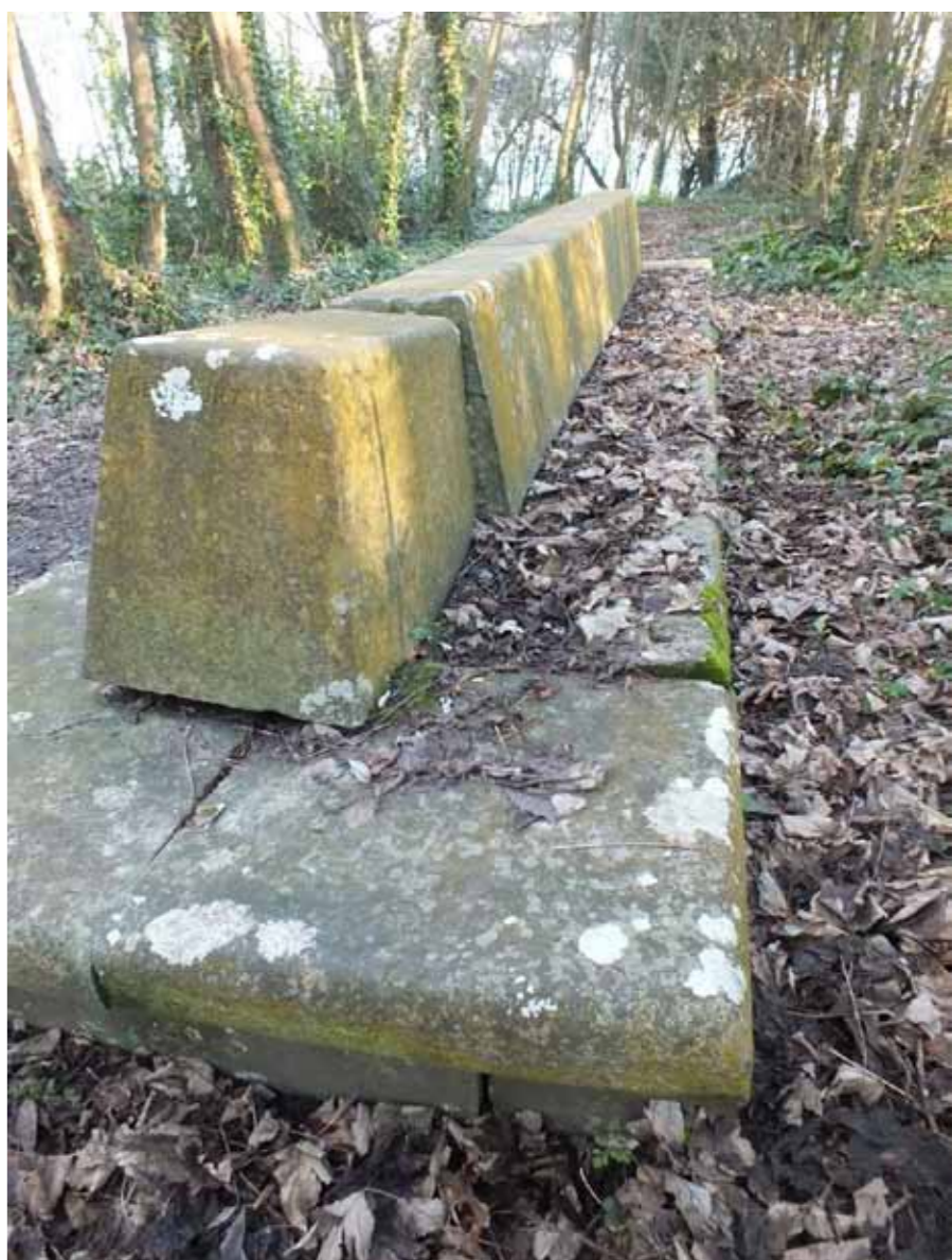
Historic Stonework (above) The historic stonework such as the lettered tablets and this 'Egyptian Seat' all need to be restored
